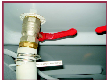
Waste water tank discharge valve
