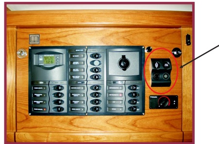
1. Bilge pump panel
