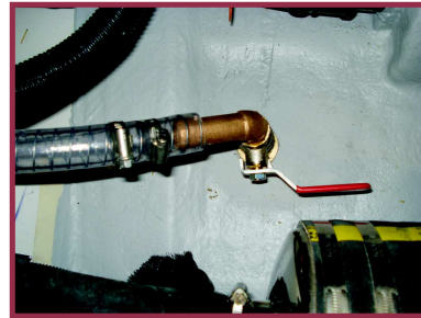
1.2. Propeller shaft engine water inlet hole with valve.
