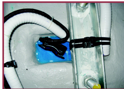
3. Bilge pump suction pipe and sensor
