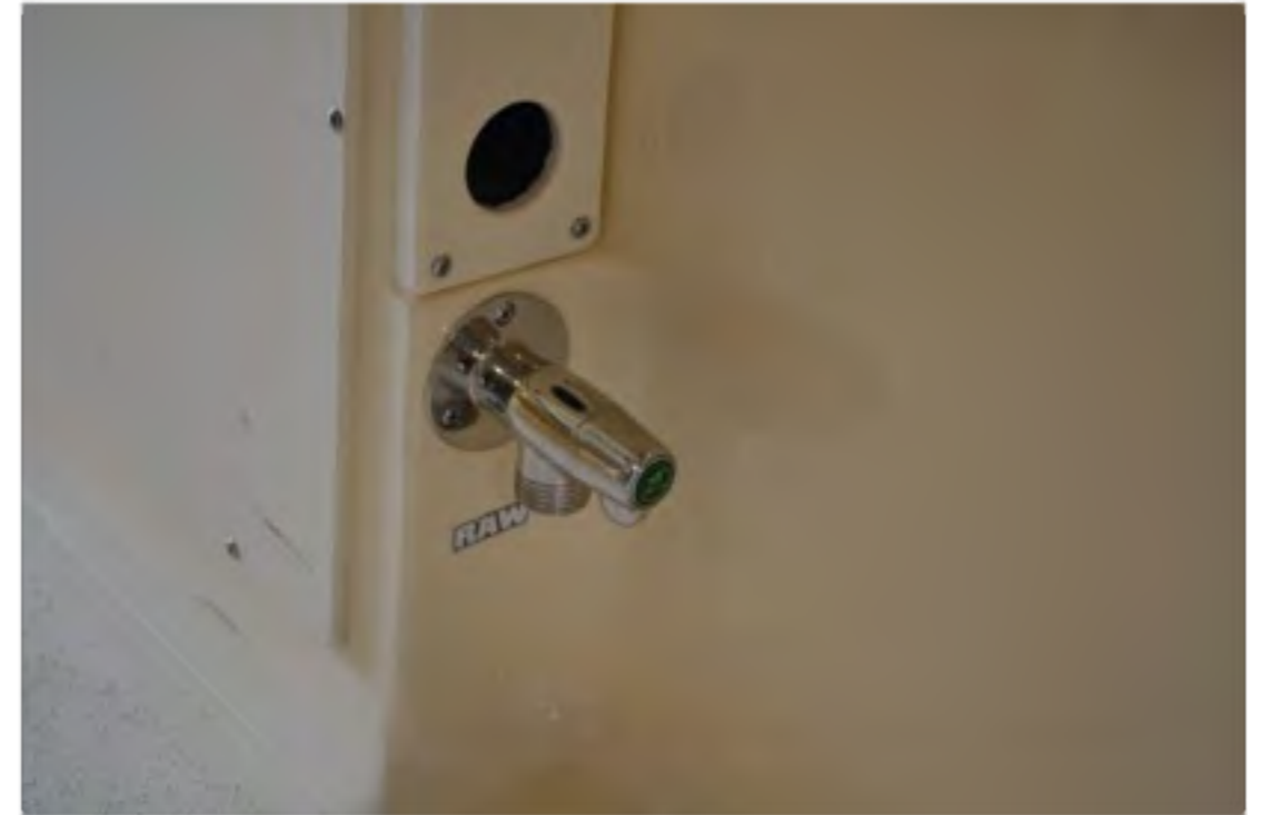
Raw Water Outlet
