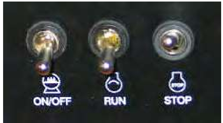
TYPICAL GEN-SET SWITCH CLUSTER- MAIN PANEL
