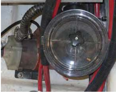
TYPICAL A/C SEAWATER STRAINER/BASKET
