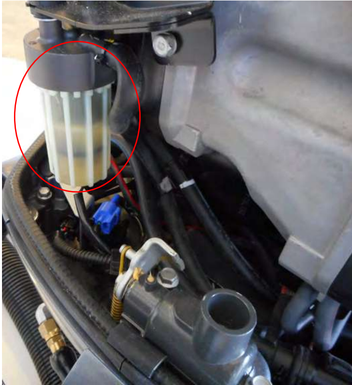
CHECKING ENGINE MOUNTED FUEL FILTER
