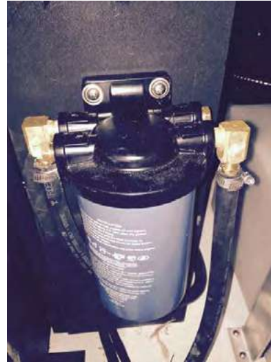
CHECKING IN-LINE WATER SEPARATOR FILTER
