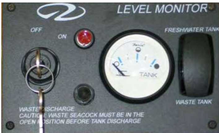
TYPICAL WATER/WASTE MONITOR PANEL
