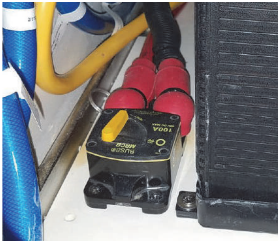
Main Battery Disconnect
