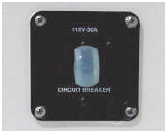
Shore Power Breaker
