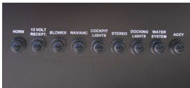
Helm Accessory Circuit Breaker Panel 214SS/218SS & 234SS/238SS
