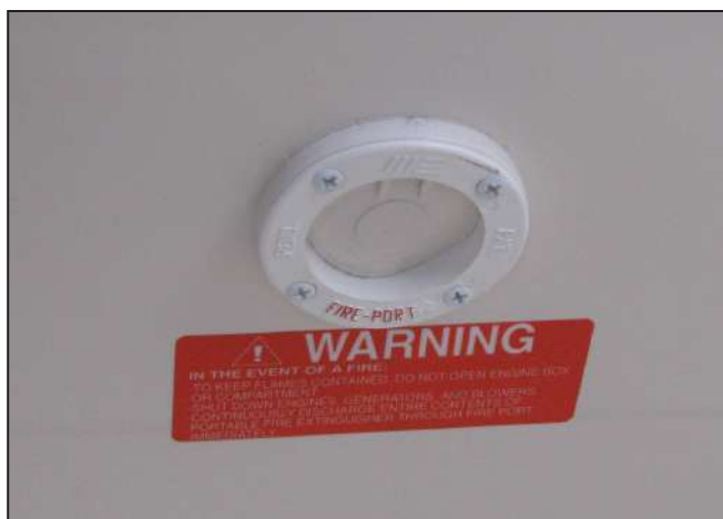
Typical Fire Port
