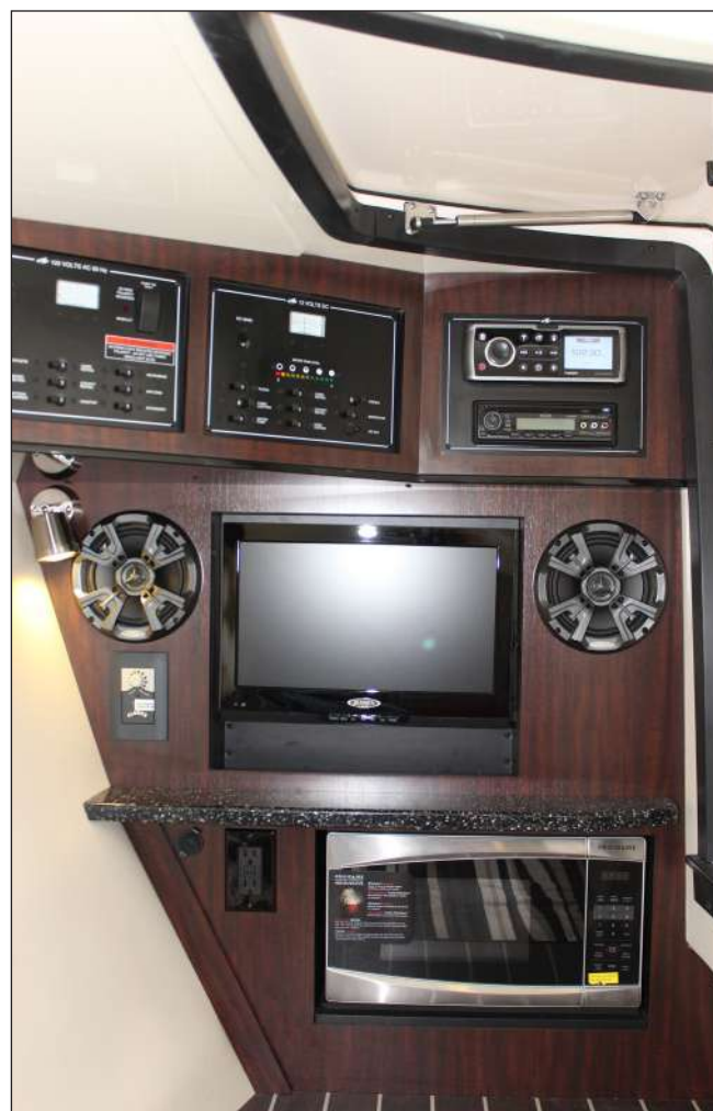
AC/DC Panels, Entertainment Center, Antenna Gain Control Panel & Microwave
