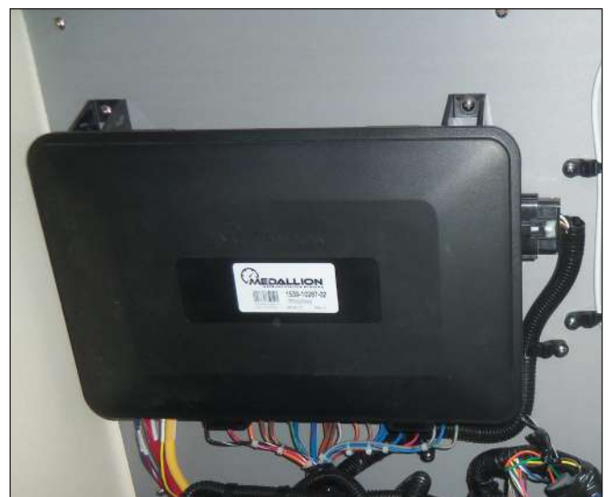
Power Management Module with Cover On
