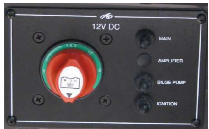
Battery Switch & Circuit Breaker Panel 214SS/218SS,234SS/238SS & 268SS
