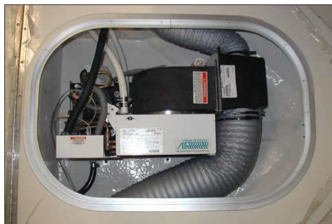
Typical 120-Volt Air Conditioner Below Berth
