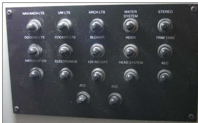
268SS Helm Accessory Circuit Breaker Panel
