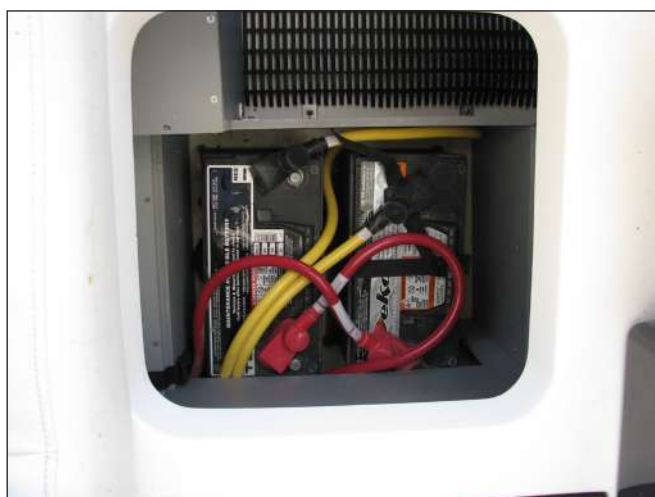
288SS Batteries In Aft Bench Seat Compartment
