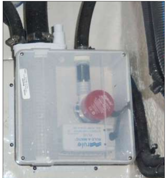
Sump Pump System
