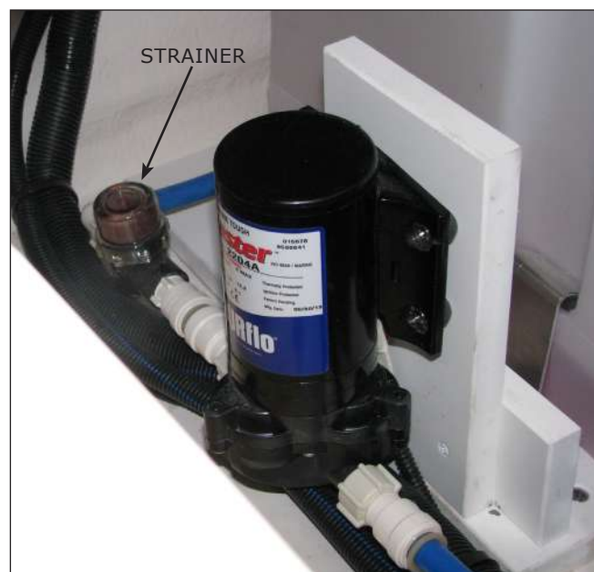
Typical Water Pump & Strainer
