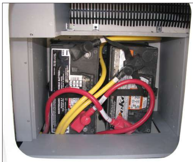
288SS Battery Installation Below Port Stern Seat
