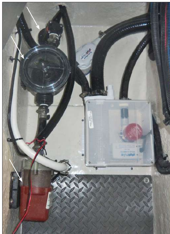
Air Conditioner Pump, Strainer & Thru-Hull Valve
