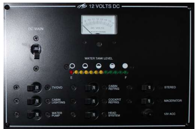
Cabin DC Electrical Panel
