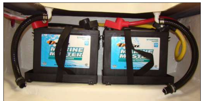
Typical Dual Battery Installation In Cockpit Storage Compartment 214SS/218SS & 234SS/238SS
