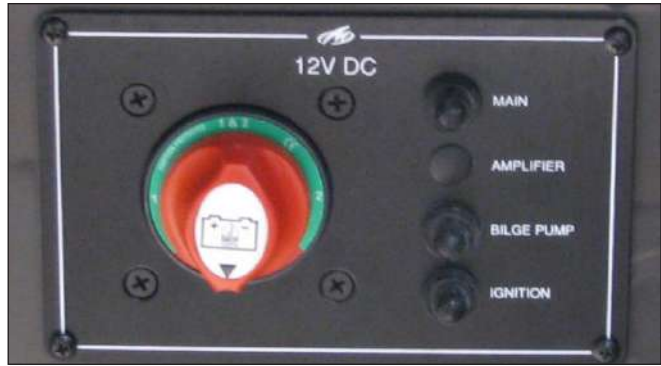
Typical 268SS Dual Battery Switch Panel
