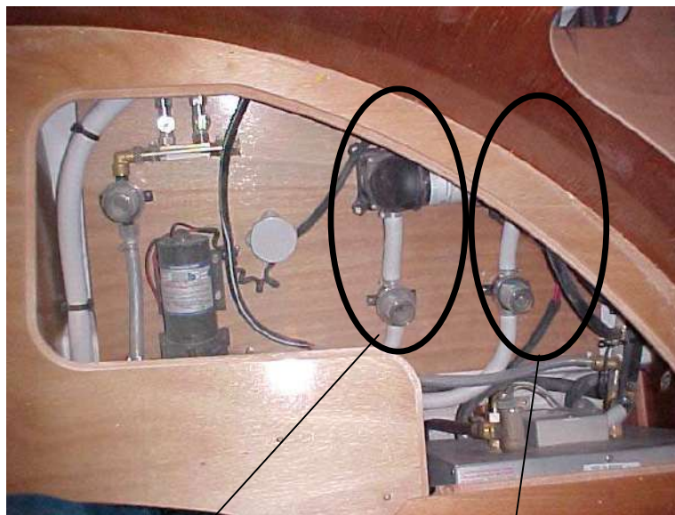
PUMP STATION UNDER STBD SETTE
